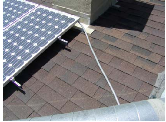
Figure 6 (incorrect) Flex conduit run without support
