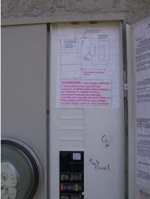
Figure 13 Sign at service entrance required by 702.8
