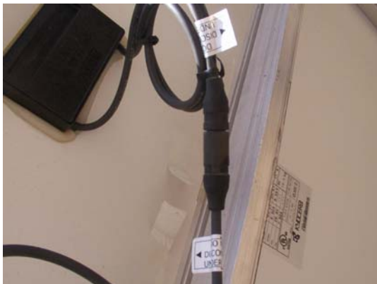
Figure 7 (incorrect) Connector loose and not supported on frame
